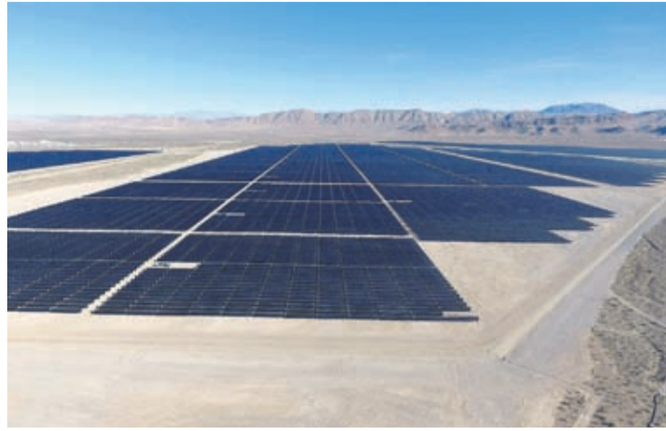
In this Dec. 11, 2017, file photo, solar arrays line the desert floor of the Dry Lake Solar Energy Zone as part of the 179 megawatt Switch Station 1 and Switch Station 2 Solar Projects north of Las Vegas.
